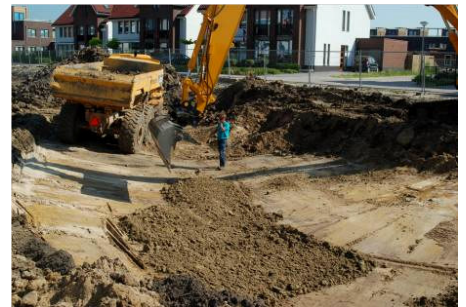
Application of the Trisoplast at the bottom of the future water garden.
