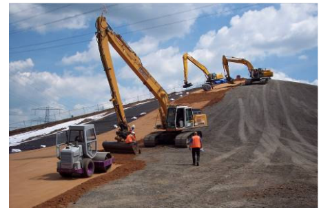
Application and compaction of Trisoplast, on not too steep slopes done by roller..
