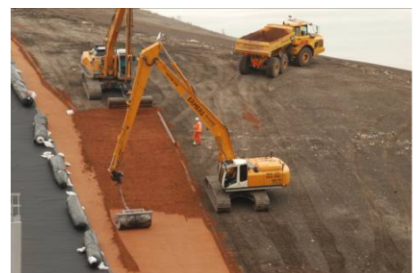
On steep slopes compaction is done using a roll attached to a crane.
