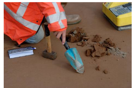
Quality control of the compacted Trisoplast layer done by an independent institute.
