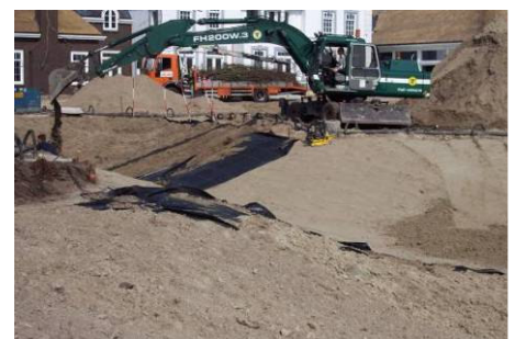
The Trisoplast layer is covered by a geotextile and a layer of loamy sand.
